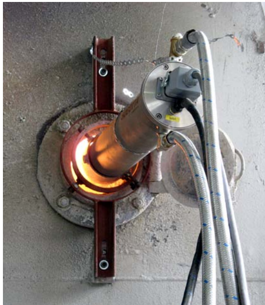
Fig. 9: IR-imager inserted through the cement kiln hood wall
